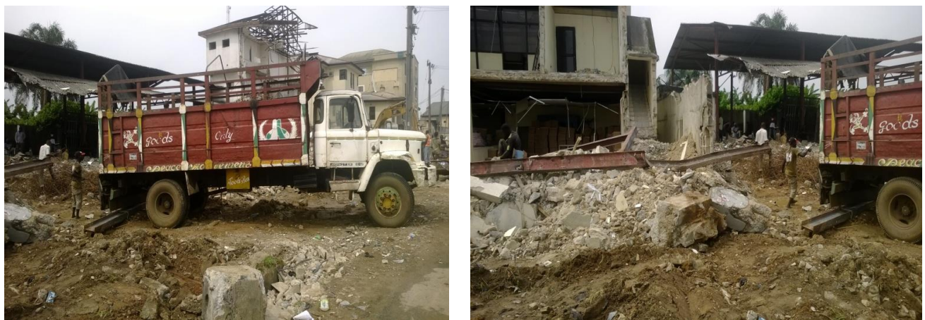
Figure 2: Pictures showing transportation of demolition waste from site at Trans-Amadi, Port Harcourt, Nigeria.
